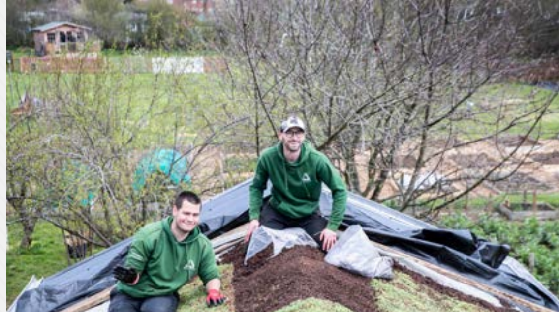
A green roof was installed to address water logging of the site
